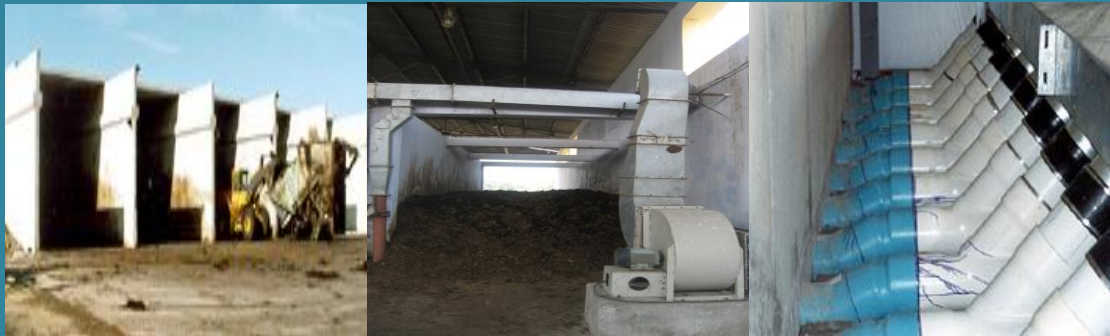
Fig.18: Bunkers and ventilation systems
