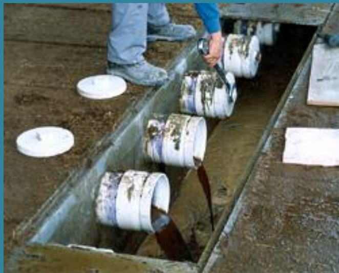
Fig.11. Under stack aeration ducts
