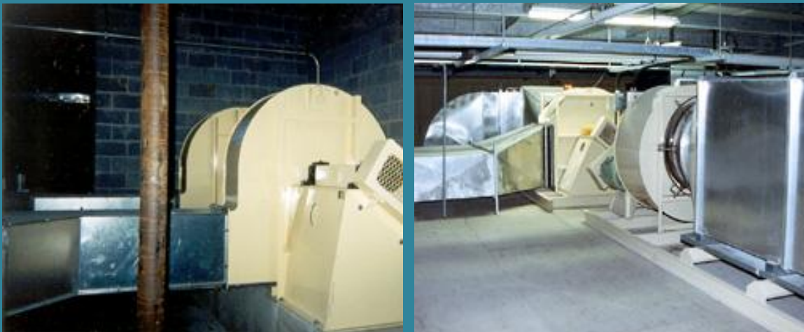
Fig.8: Tunnel with air handling unit
