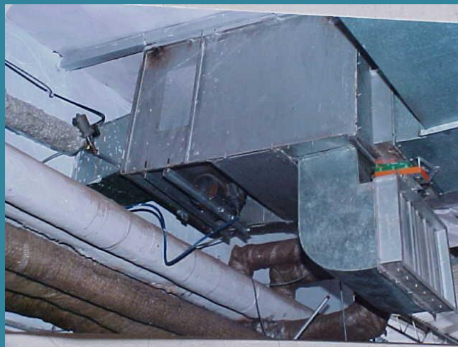
Fig.13. A standard AHU with centrifugal Blower
